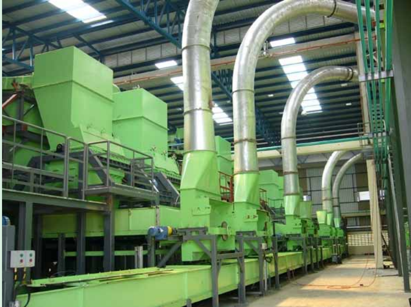
RDF processing system in Malaysia
