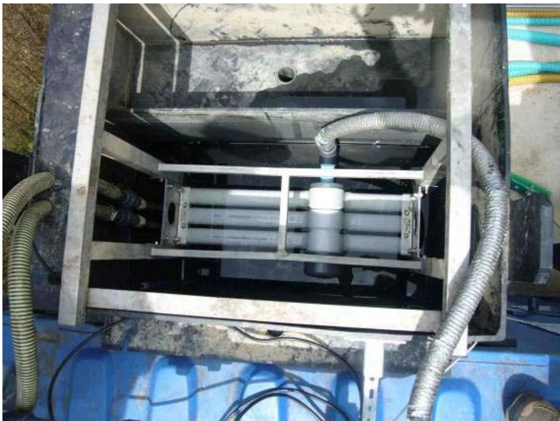
Figure 4. UV radiation unit for post disinfection of reclaimed wastewater for irrigation
