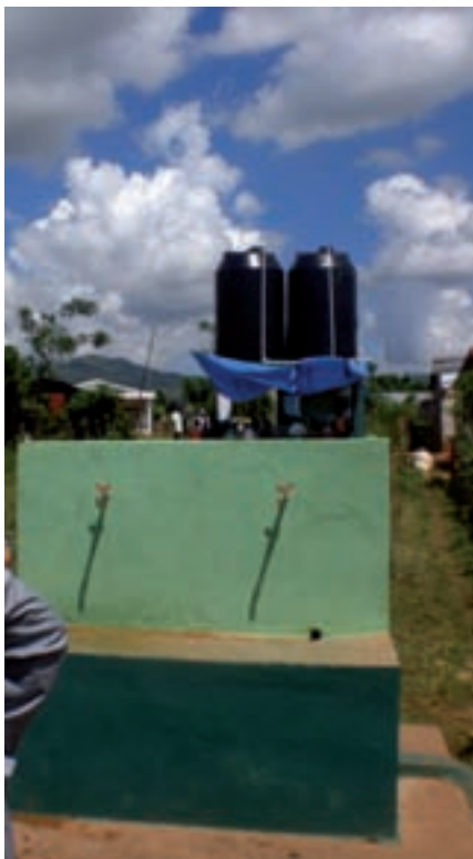
Fig. 10. Inauguration of a supply source in Monte Plata (Dominican Republic). Action sponsored by the WCCE and developed by CEZOPAS and the Spanish Cooperation Fund for Water and Sanitation (FCAS).
