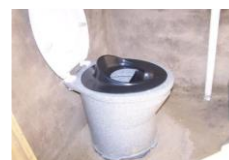
Urine diversion toilets
