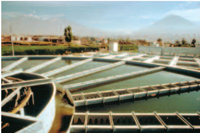
Fig. 8. Peru water treatment plant. Source: WHO.
