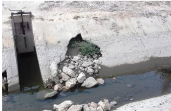
Damage in mesqas lining (Photo 8)
